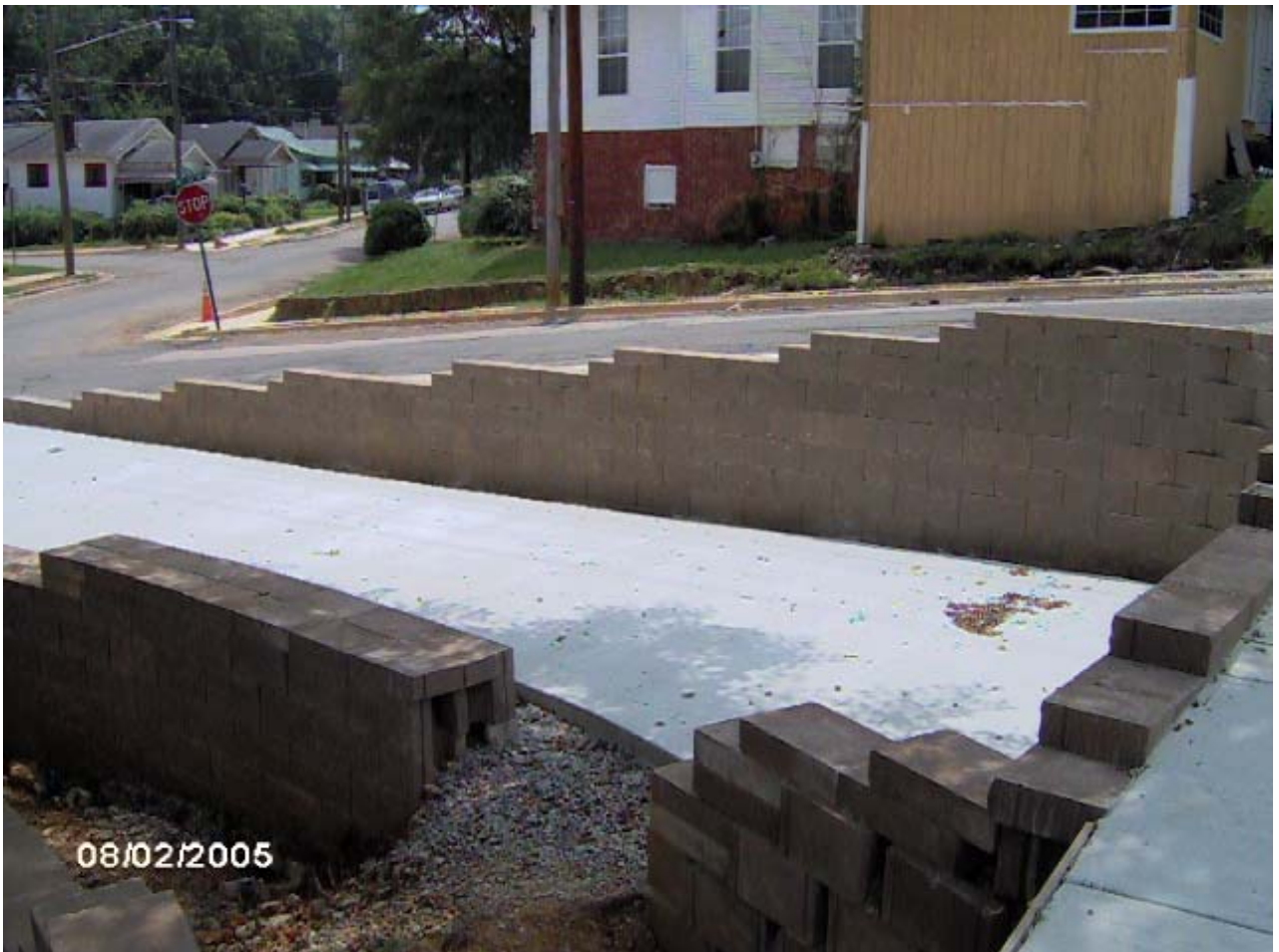
TUXEDO COURT CONSTRUCTION PROGRESS AT THE NORTHERN TRIANGLE IN THE FOUNTAIN HEIGHTS NEIGHBORHOOD
