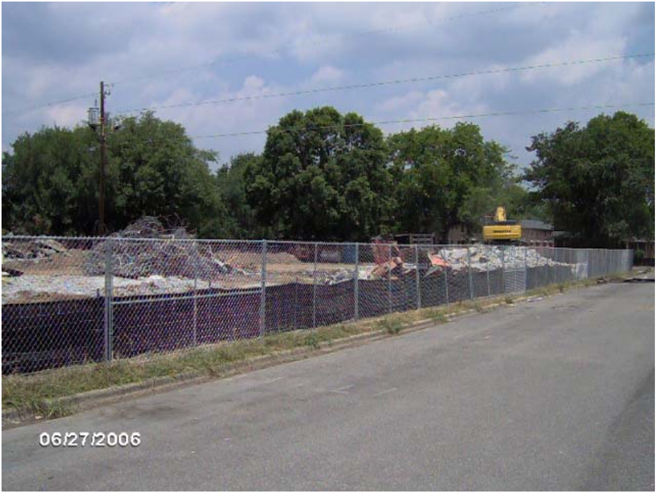
TUXEDO COURT DEMOLITION SERVICES ON BLOCK 9 AT TUXEDO COURT PHOTOGRAPH TAKEN TUESDAY, JUNE 27, 2006
