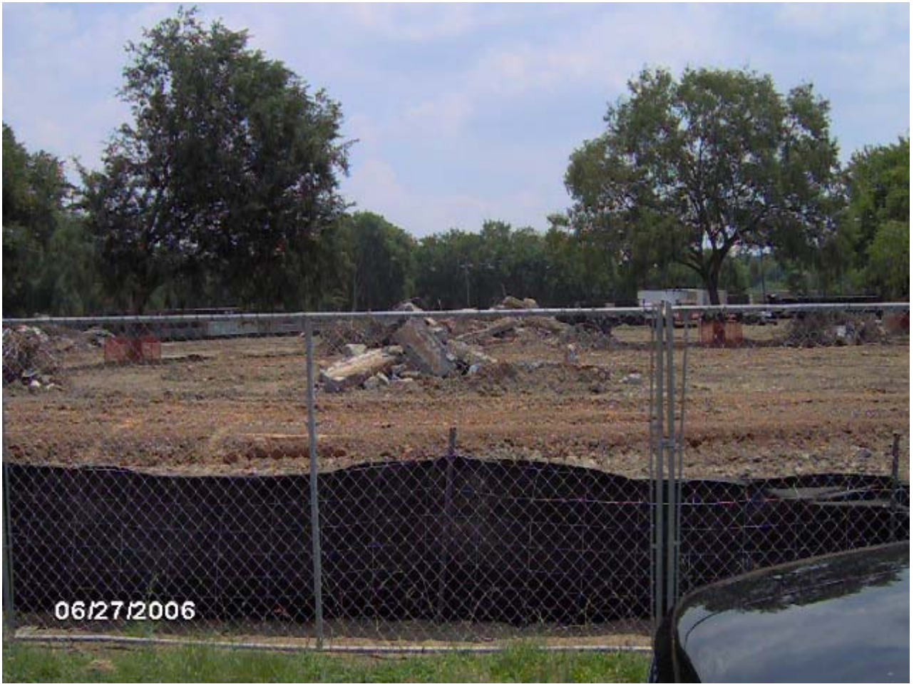
TUXEDO COURT DEMOLITION SERVICES ON BLOCK 10 AT TUXEDO COURT PHOTOGRAPH TAKEN TUESDAY, JUNE 27, 2006
