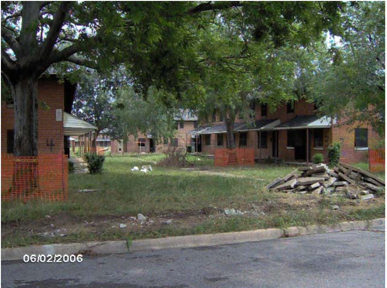
TUXEDO COURT DEMOLITION SERVICES ON BLOCK 10 AT TUXEDO COURT PHOTOGRAPH TAKEN FRIDAY, JUNE 2, 2006
