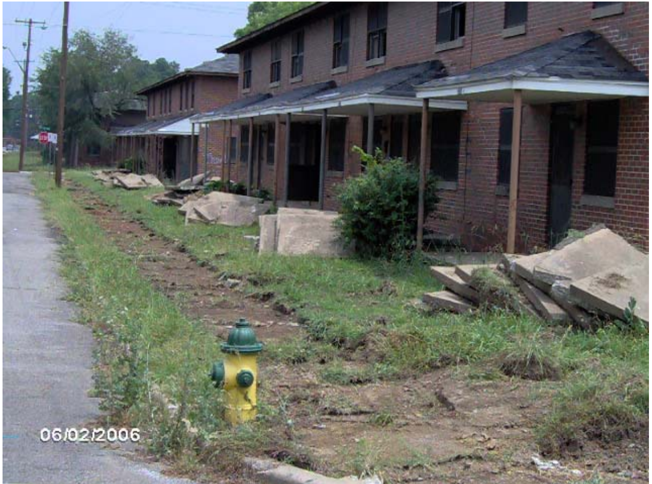
TUXEDO COURT DEMOLITION SERVICES ON BLOCK 9 AT TUXEDO COURT PHOTOGRAPH TAKEN FRIDAY, JUNE 2, 2006
