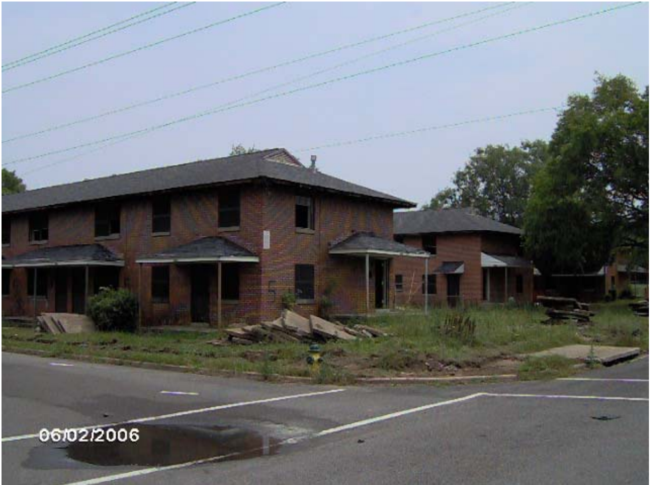
TUXEDO COURT DEMOLITION SERVICES ON BLOCK 10 AT TUXEDO COURT PHOTOGRAPH TAKEN FRIDAY, JUNE 2, 2006
