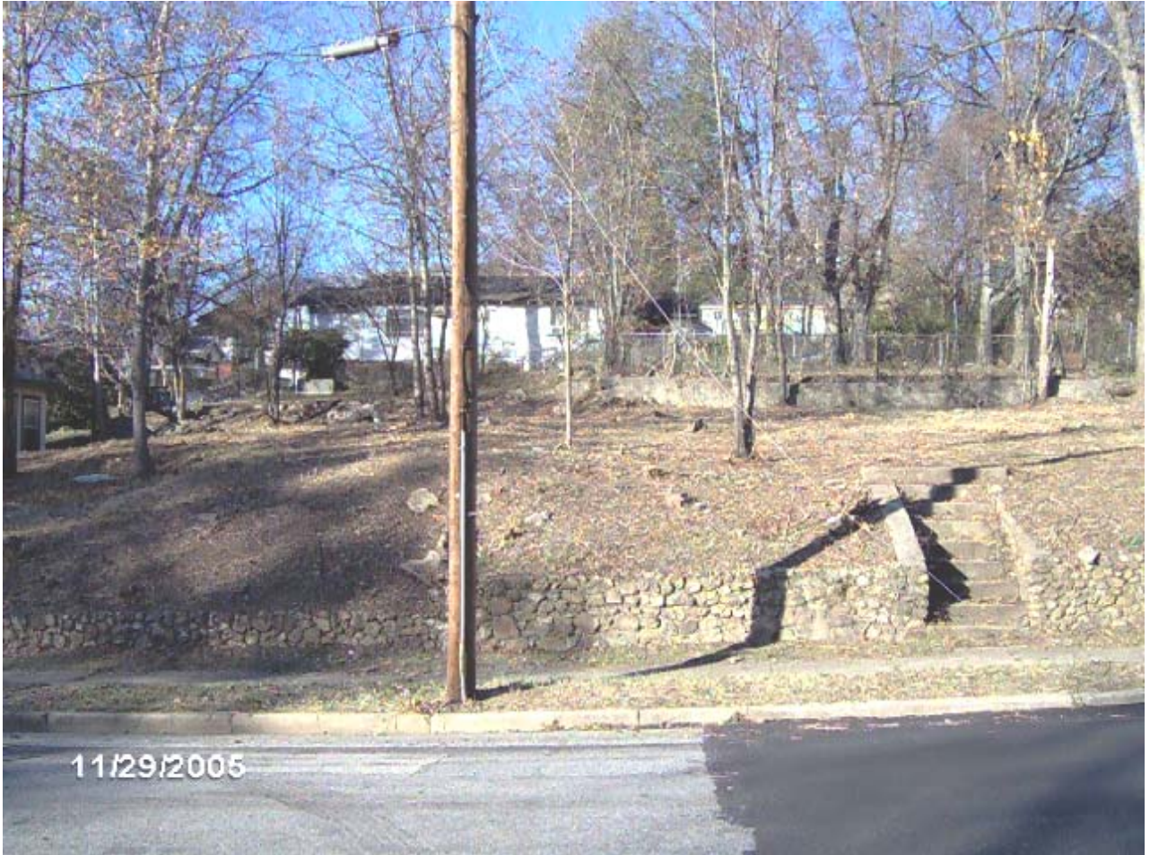
TUXEDO COURT CLEARING LOTS FOR HOME CONSTRUCTION PREPARATION IN THE FOUNTAIN HEIGHTS NEIGHBORHOOD
