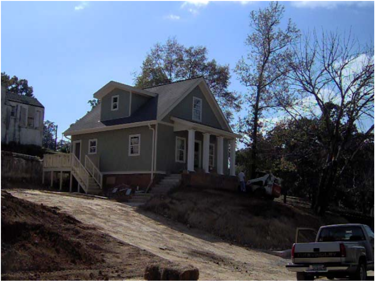
TUXEDO COURT LOT 2 ALONG 15 TH AVENUE NORTH IN FOUNTAIN HEIGHTS FINAL GRADING OF FRONT YARD
