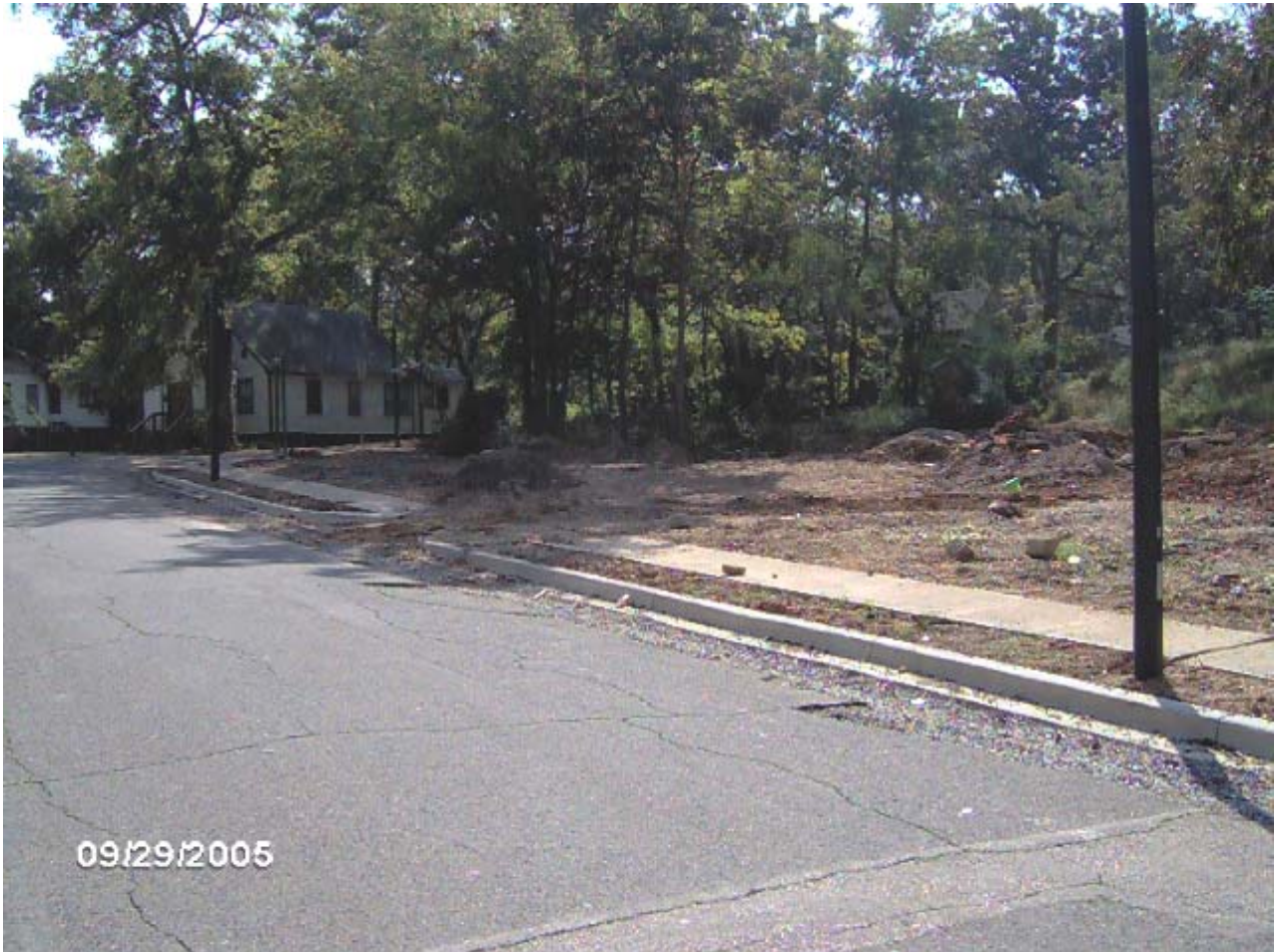
TUXEDO COURT PEDESTRIAN LIGHTING BEING INSTALLED ALONG 15 TH AVENUE NORTH IN THE FOUNTAIN HEIGHTS NEIGHBORHOOD
