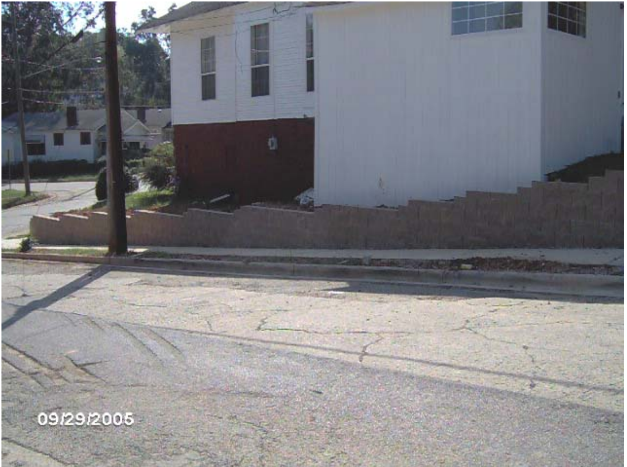
TUXEDO COURT NEW RETAINING WALL SOUTH OF THE NORTHERN TRIANGLE IN THE FOUNTAIN HEIGHTS NEIGHBORHOOD
